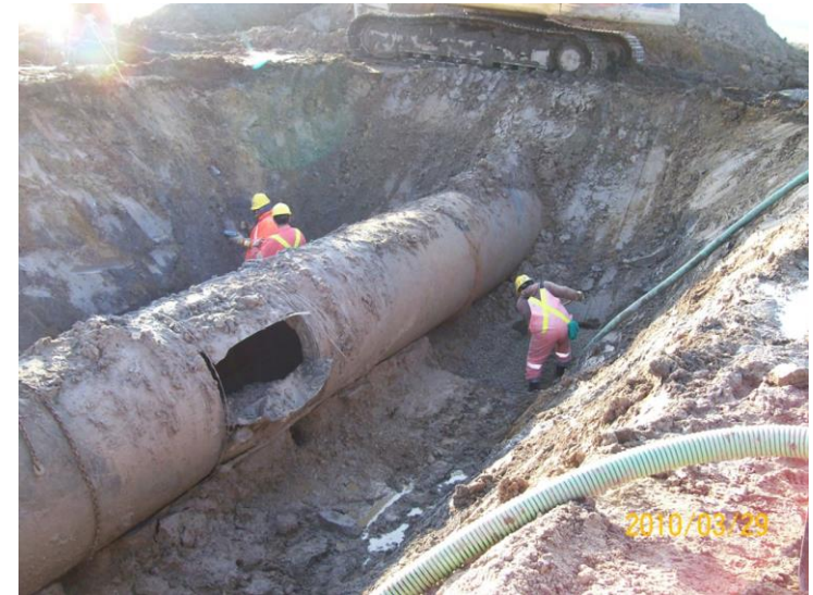
Reported Leaks (surfacing)
