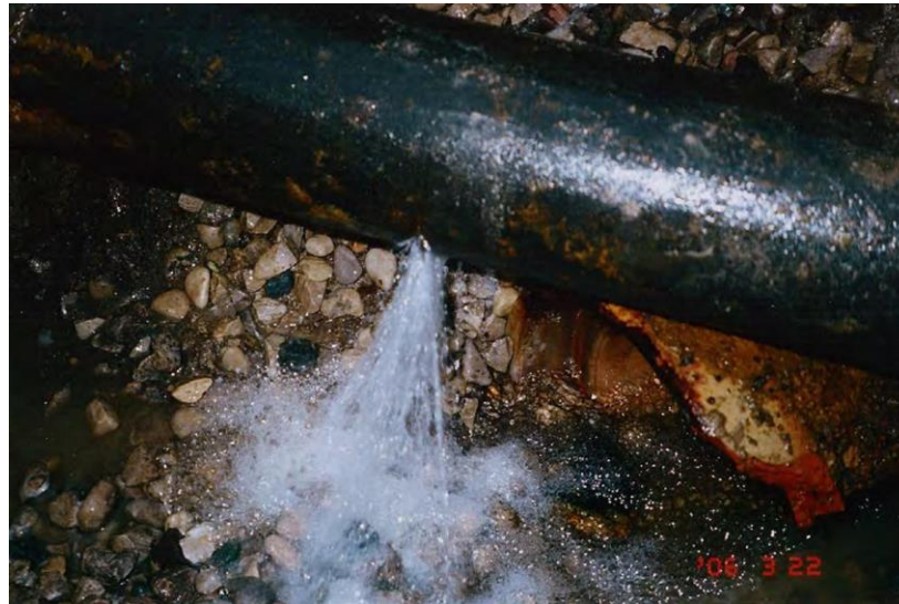
Unreported Leaks (not surfacing)
