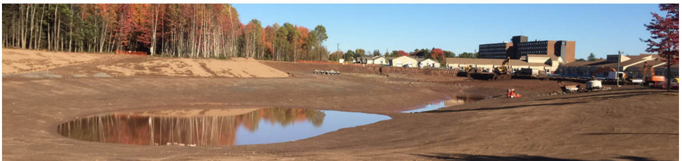
A naturalized stormwater retention pond (City of Moncton) that can evolve to provide natural infrastructure benefits. Photo ©Ducks Unlimited Canada. Used with permission.
